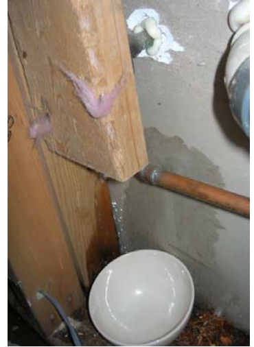
Supply Leak & Damage
